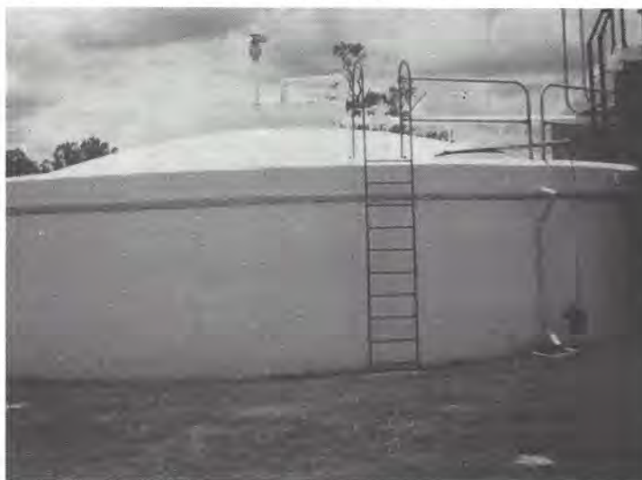
Fig 3.14: Sewage digester (sludge treatment).
